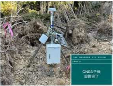
GNSS子機G-1 (23/10/27設置)
